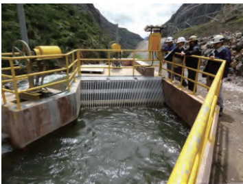
Hydroelectric power plant in Huanzala Mine, Peru
